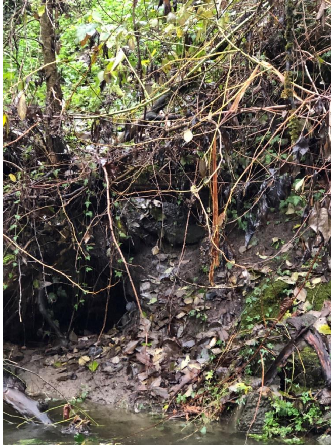
Figure 2-15: Signs of erosion downstream of I-405
