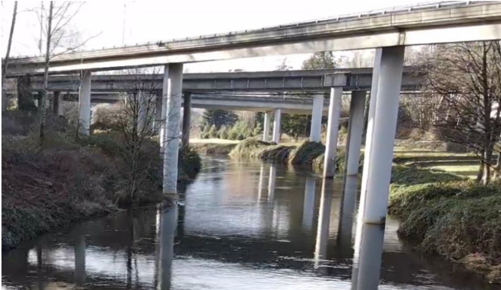
Figure 4. Photo of the Sammamish River looking west through the crossings. Note the right bank scour around the existing NB I-405 to WB SR 522 bridge column in the foreground (January 1, 2023 site visit).
