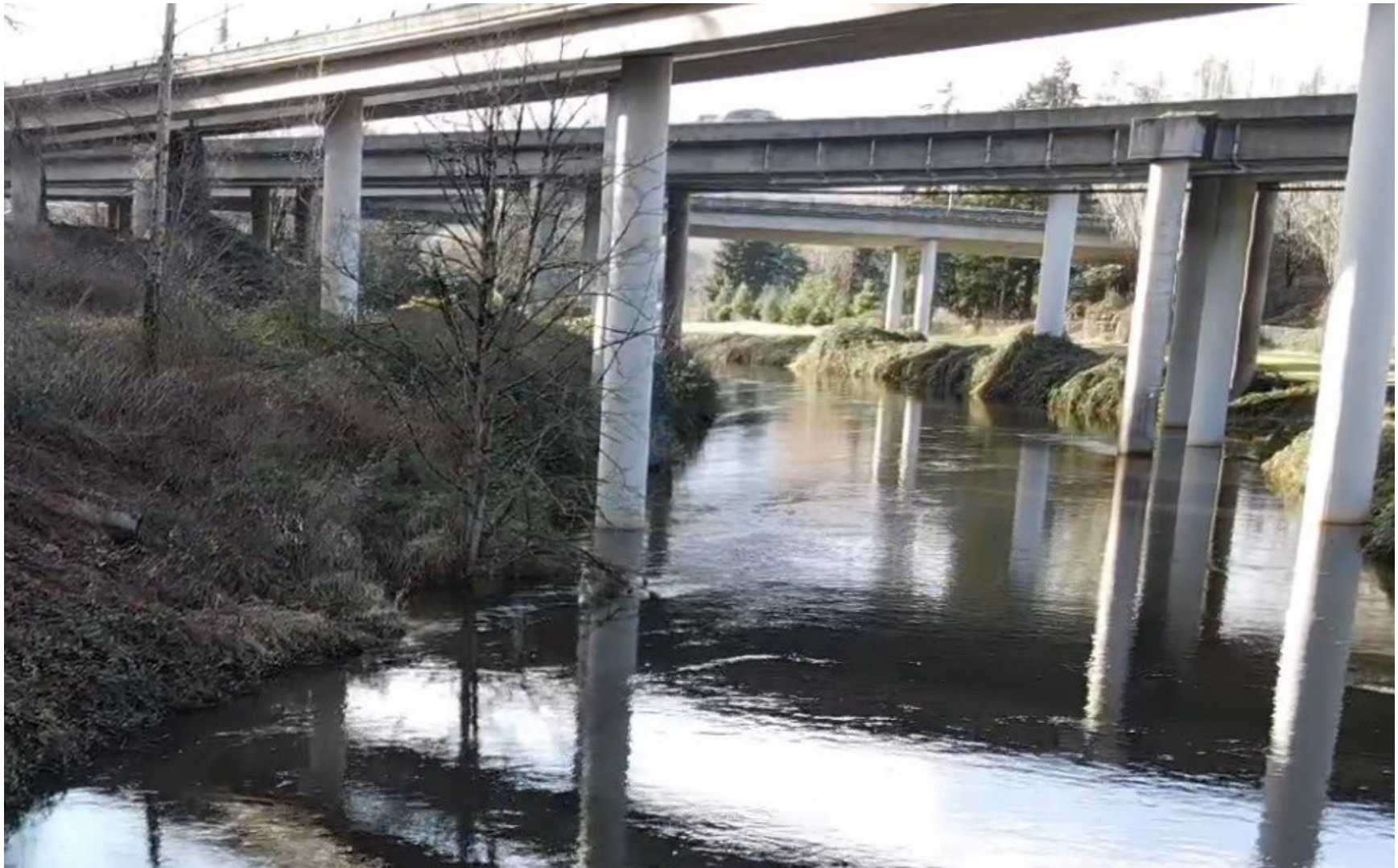
Figure 5. Photo of the Sammamish River looking west through the crossings. Note the right bank scour around the existing NB I-405 mainline bridge columns (January 1, 2023 site visit).
