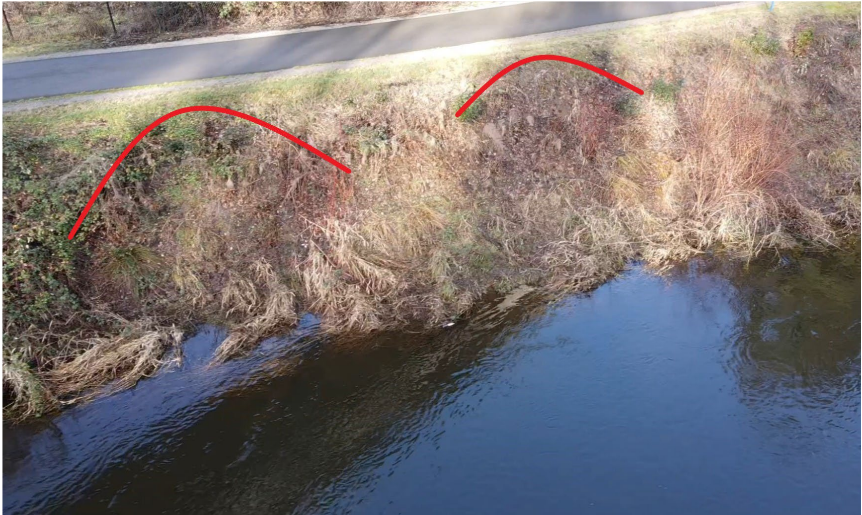
Figure 3. Photo of north bank sloughing at 20 feet and 60 feet north of the existing NB I-405 to WB SR 522 bridge crossing (western end of the King County repairs) taken during January 1, 2023 site visit. The red lines highlight the top of impacted bank slope.
